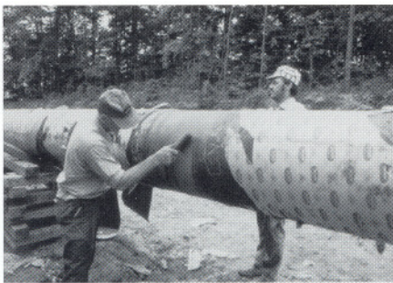
Pipe surface is wire brushed to remove loose scale, rust and dirt.
