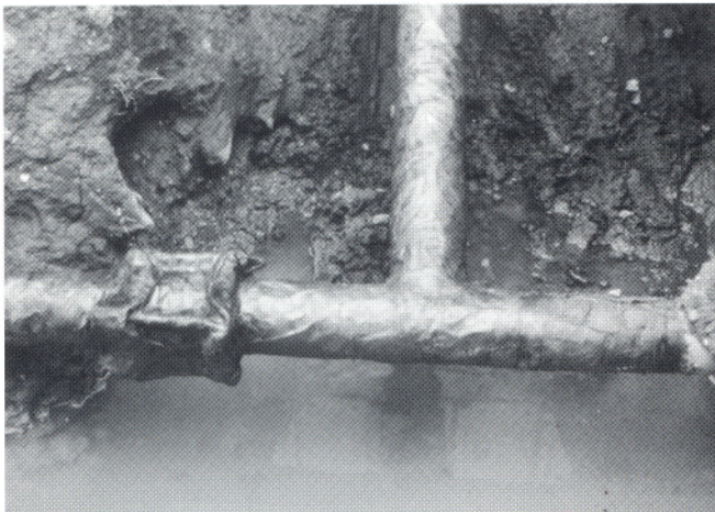
Completed application of Graycoat® and Guard-Wrap to welded tee and 4-bolt compression coupling.
